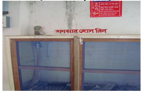
[Fire Hose Pipe/Reel]
